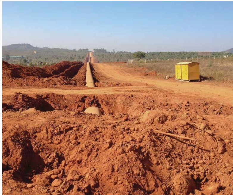
China's Shwe Gas pipeline in Myanmar.
