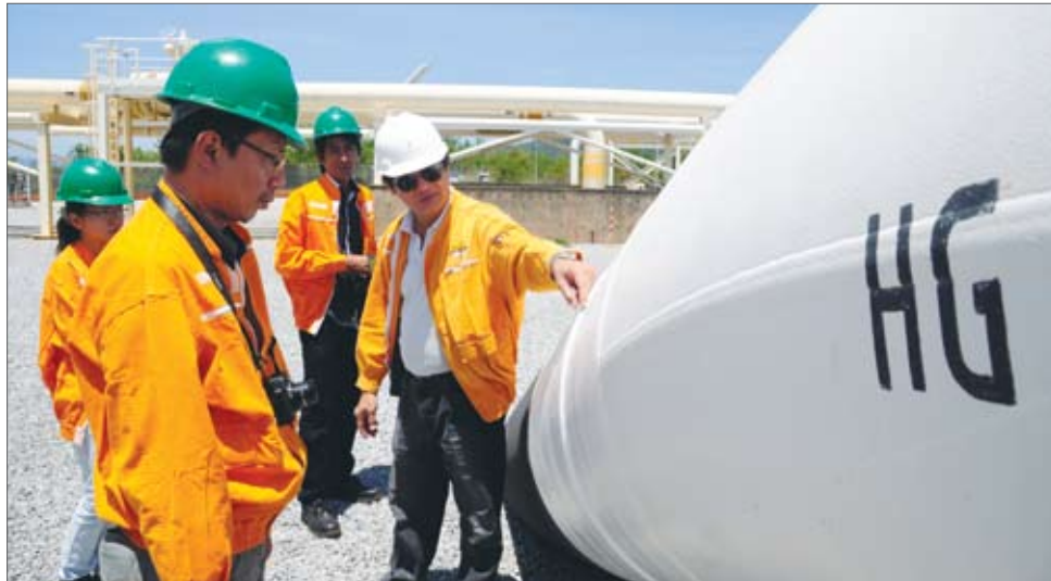
An engineer explains about the gas pipeline to journalists at Kanpauk in southern Myanmar last year. PIC: THE MYANMAR TIMES
